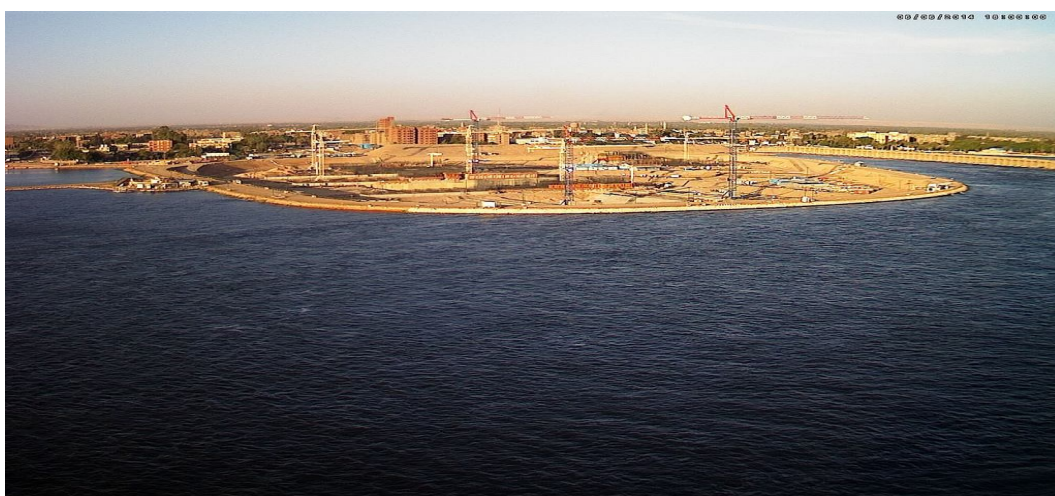
Figure (2): The construction pit for the New Assuit Barrage and Hydropower Plant
